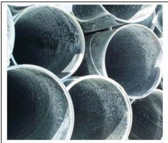
Light white rust formed inside large diameter galvanized pipes caused by prolonged period of wetness after galvanizing and slow drying of the shaded sections of the pipes.
