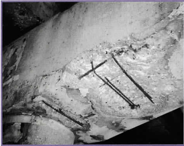
Carbonation induced corrosion on road bridge deck beam
