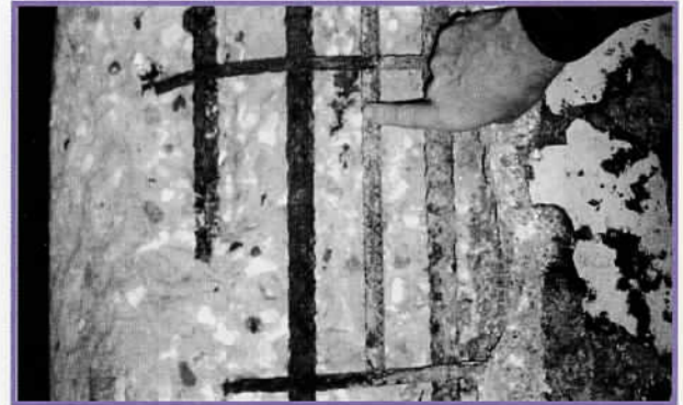
Chloride induced rebar corrosion on bridge column.
