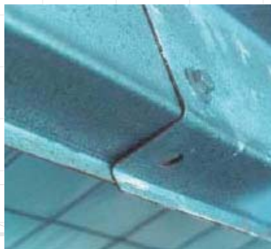
Pre-galvanized products rely on cathodic protection to prevent corrosion on their cut edges. Thicker sections such as these heavy purlins are on the borderline and corrosion is visible on installation.
