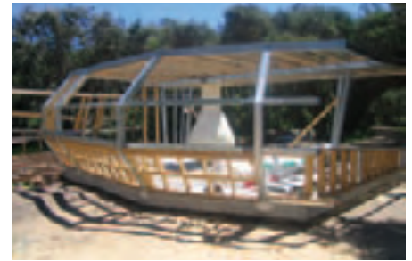
The angled planes of the bedroom wing walls were enabled by steel wall beams and cranked circular hollow section columns.
