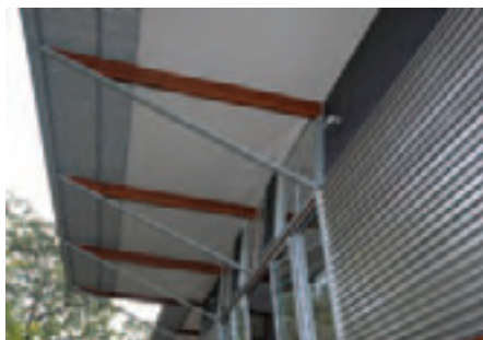
The roof has ventilation slots to allow convection cooling to the roof cavity.
