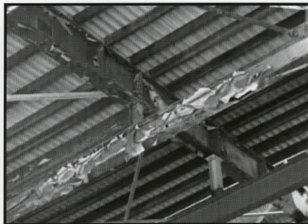
These crane monorail beams are being refurbished in the pre-treatment area of a galvanizing plant, where the original epoxy coating has failed completely. The beam at the rear has been removed, abrasive blasted, hot dip galvanized and coated with an acid-resistant chlorinated rubber paint coating.
