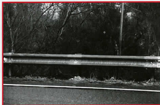
This section of galvanized guardrail has been subjected to a recent Australian bushfire. Although smoke stained & discoloured, the coating is still in excellent condition.
