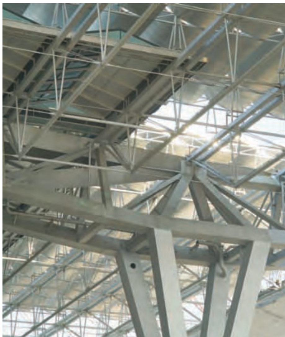
Partially complete, the installation of the skylight and louvre modules progresses above the super truss steelwork.
