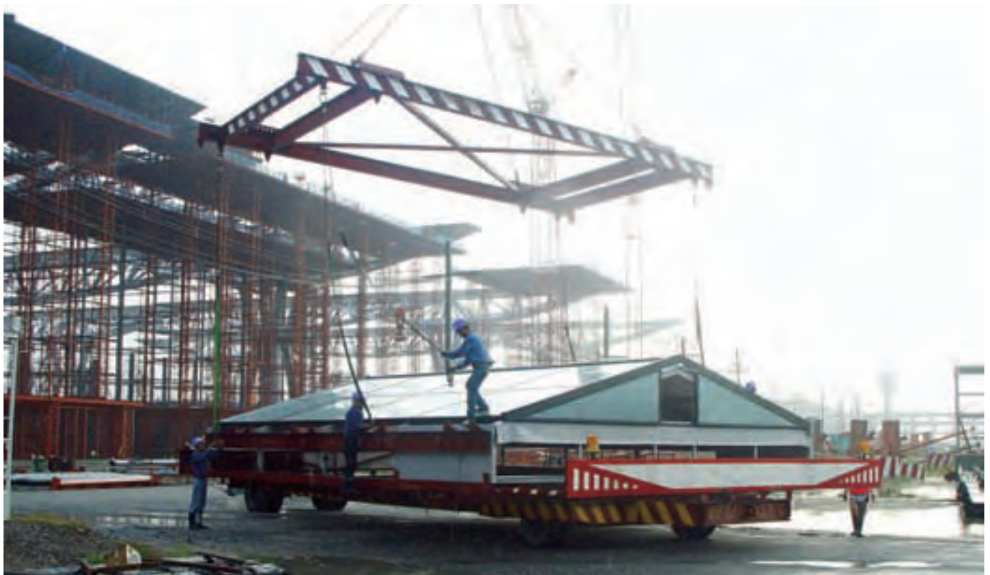
Gable end skylights were pre-assembled, complete with glazing, cladding and water proof membrane, ready for erection.
