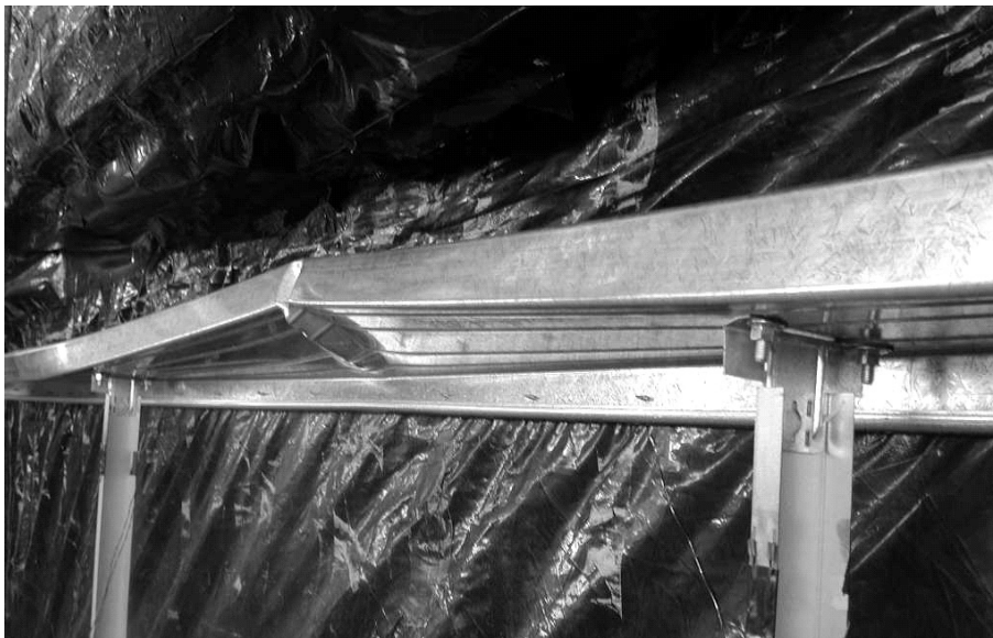
Fig. 5.17 Bridging bolted to purlin (failure under test between bridging points)
