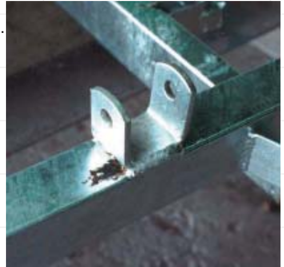
Blow-out from over lapping area on this fabrication has caused a galvanized coating defect
