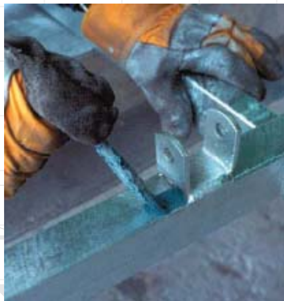
Approved epoxy-based zinc-rich paint is applied to the uncoated area to at least equivalent thickness to the galvanized coating.
