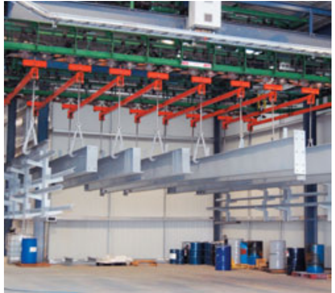
The monorail that services the advanced new paint line at Ahrens.
