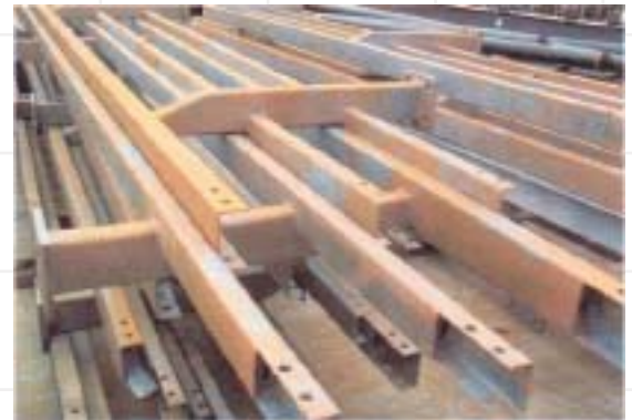
These steel bridge railings have been abrasive blasted prior to coating but have flash-rusted, requiring further surface treatment prior to coating
