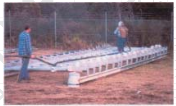
These galvanized conveyor frames are being brush-blasted prior to the application of a heavy-duty paint coating. This is a very effective surface treatment for painting over galvanized surfaces.
