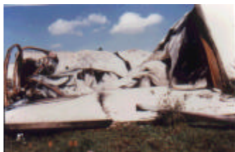
failure of connections causing external wall panels to collapse outwards during fire
