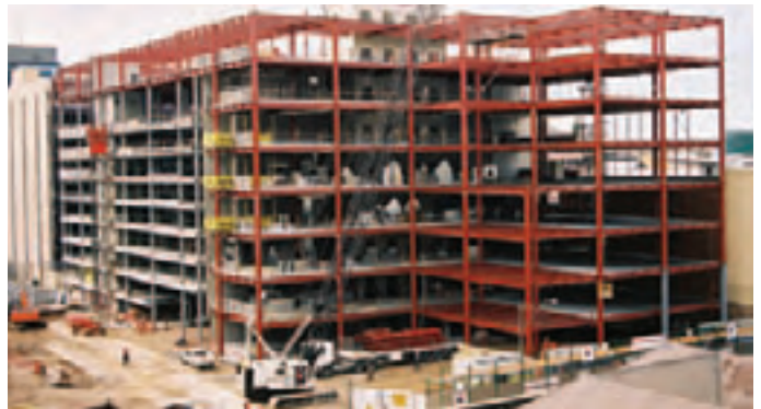
Structure during steelwork erection of stages two and five - the carpark and IAG building. The extended floors at levels seven and eight are taking shape over the carpark.
