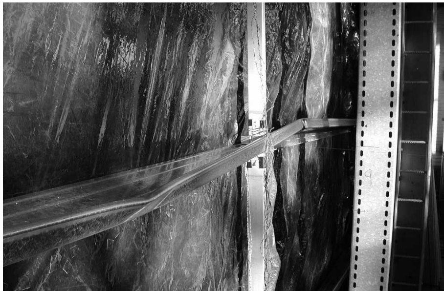
Fig. 3.13 Purlin flexural-torsional buckle with distortional buckle (foreground) and local buckle (background)
