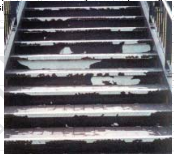
Complete failure of this paint system on this galvanized stairway occurred because the paint was applied directly to the chromate quenched galvanized surface. This passivation treatment interferes with paint adhesion
