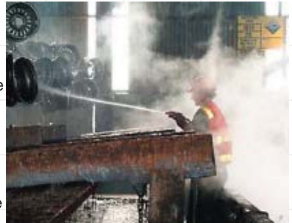
Chemical pre-treatment usually involved multiple processes. This hot caustic degreasing operation in the hot dip galvanizing process is necessary to ensure the acid pickling stage is effective.
