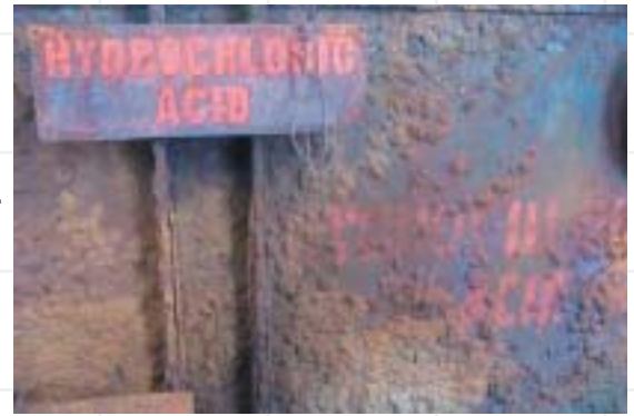
Difficult surfaces such as the corroded steel shell of the hydrochloric acid pickling tank require stringent surface preparation to remove both corrosion products and residual chlorides
