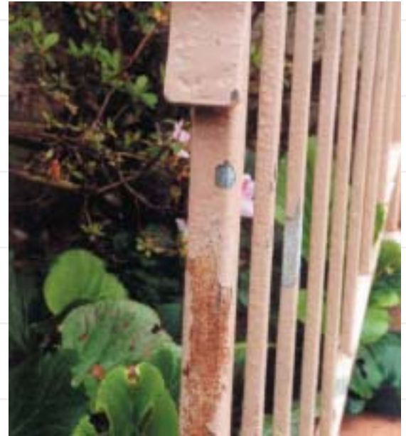
Paint failure on galvanized balustrade resulted from paint being applied to a contaminated surface.
