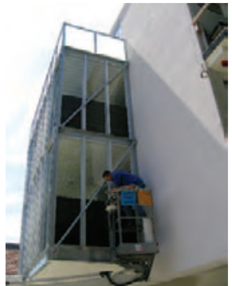
Angled tension rods form part of the add-on structure, providing additional strength and tension.
