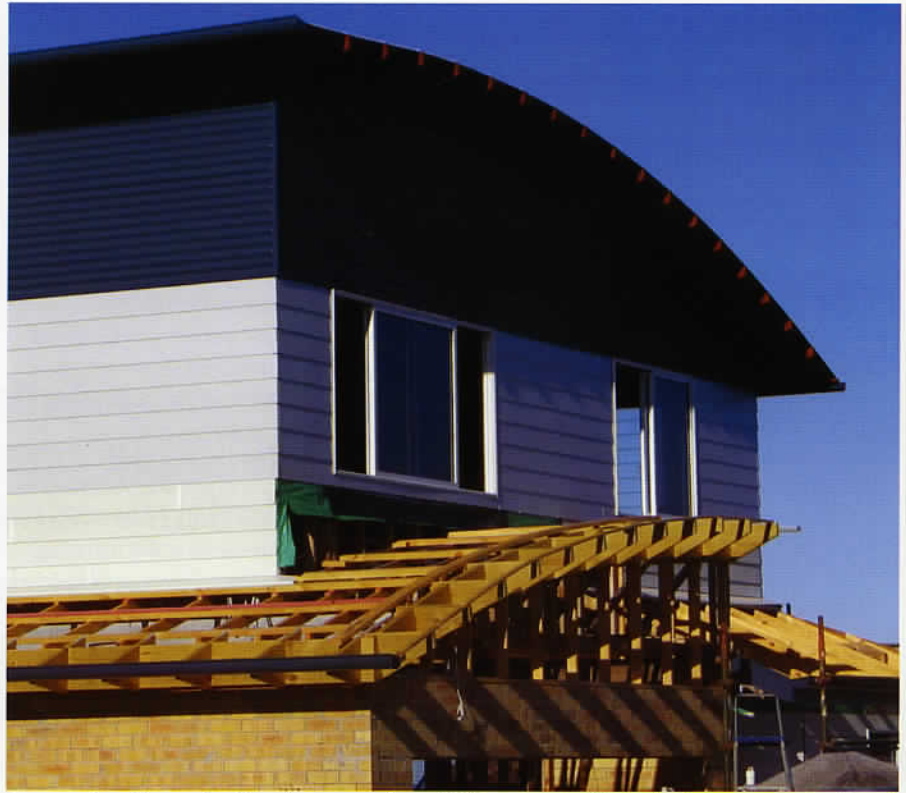
Any construction project involves a number of different materials including uncoated, painted and galvanized steel, aluminium, aluminium-zinc alloy coated steel and copper-chrome-arsenic treated timber and copper, brass or lead in lesser applications. The compatibility of these materials in contact will influence their durability.
