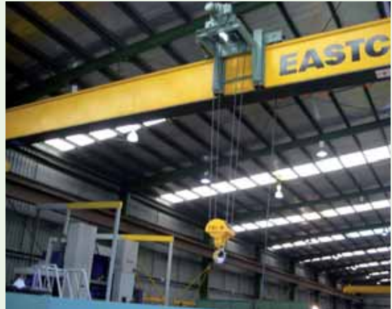
Overhead cranes must be rated to the correct SWL.
