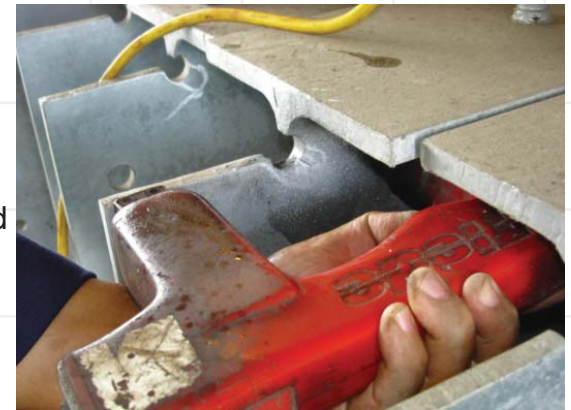
These large galvanized beams, galvanized in Malaysia, have all been affected by 'cope cracking' in the circular (coped) area of the beam webs. Steel sourced from electric furnace sources is more prone to this form of liquid metal assisted cracking than steel sourced from blast furnaces. This phenomenon has never been reported in Australia as all the locally produced structural sections are manufactured from blast furnace sources.
