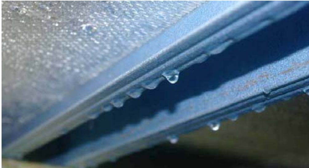
Condensation on the impermeable foil sarking and steel purlins
