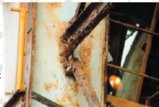
The cost of the coating materials for maintenance coating of rusting structures is insignificant compared to the cost of surface preparation, environmental management and access.
