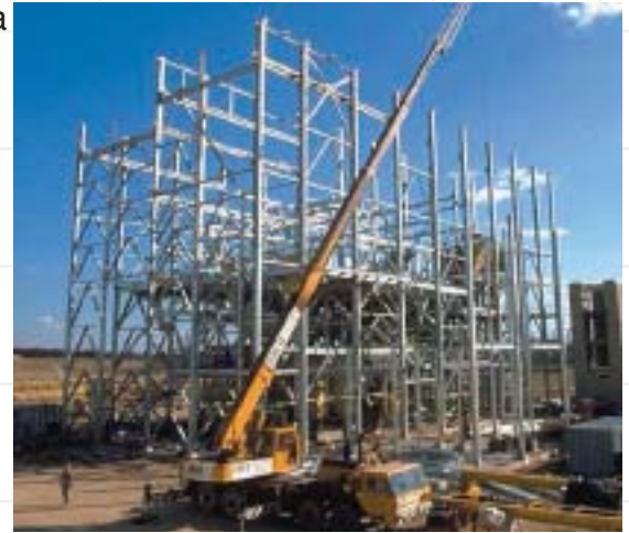
Industrial facilities like this coal treatment plant at Teralba, NSW process 800 tph of coal 24 hours/day, 7 days/week. The cost of down-time for coating maintenance is a bigger factor than coating cost.
