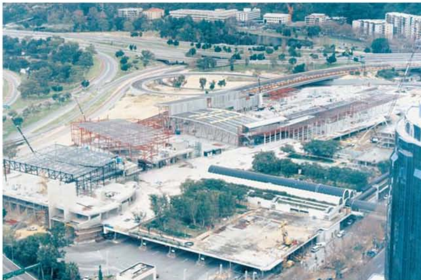
Modelled in 3D the multi million dollar Perth Convention and Exhibition Centre is taking shape on the banks of the Swan River
