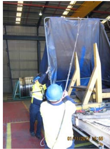
Old wet weather canopy – 2 man operation
